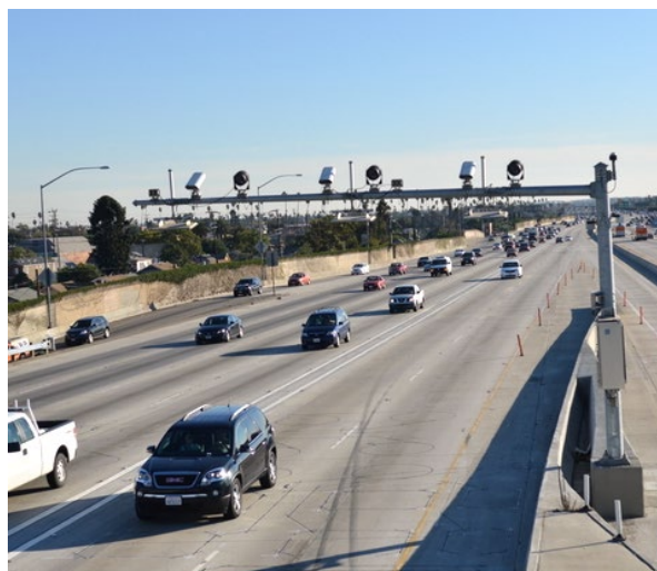
Figure 24: I-110 ExpressLanes Toll Gantry
