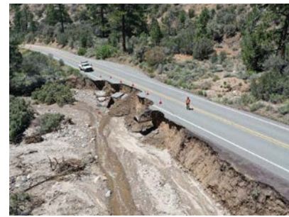
State Route 38 Storm Damage
