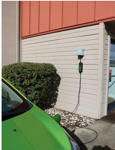
Level 2 16-Amp with NEMA 14-30 receptacle
