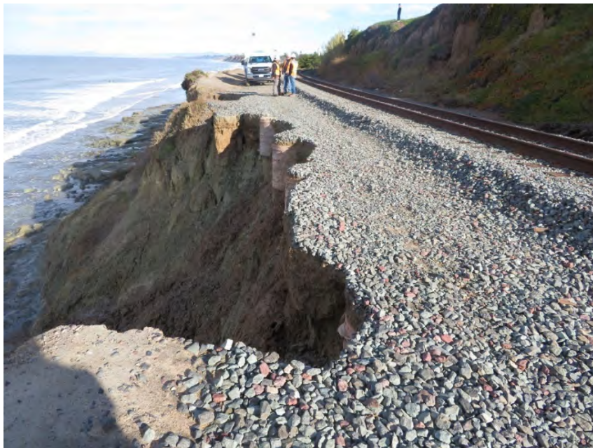
Photo 3: Bluff Slide Thanksgiving 2019 Resulting from Surface Drainage over Bluffs.
