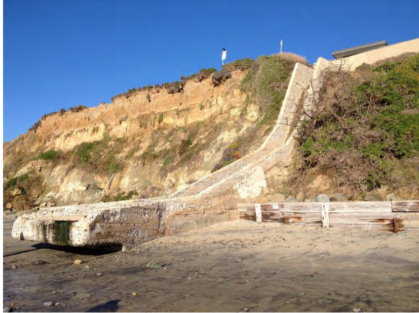
Photo 2: Aging Drainage Structure to be Replaced.
