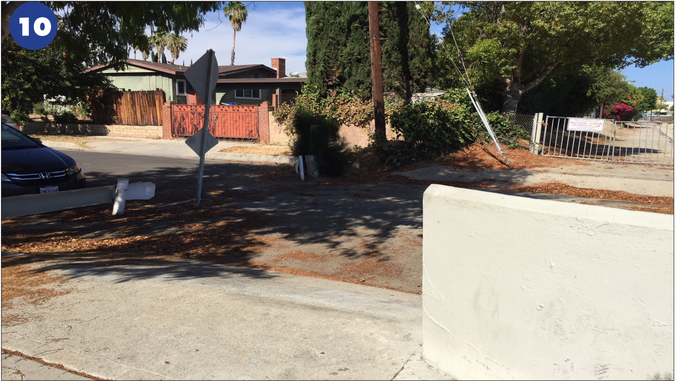
Amigo Street, north bank of LA River. Note non ADA-compliant ramp.
