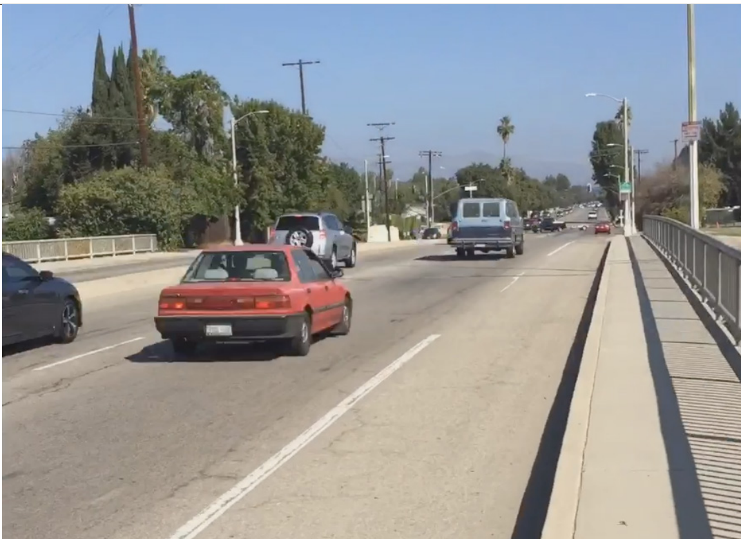
Unimproved Project Area - Existing White Oak Ave bridge over L.A. River with Class II bikeway - Looking north. Note poor paint quality and lack of protection; note narrow sidewalk and wide auto travel lanes.
