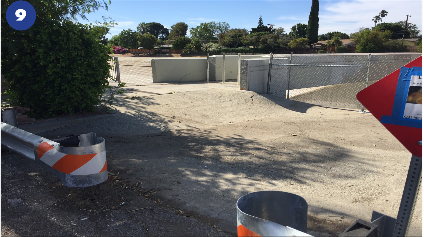
Amigo Street end, south bank looking north at pedestrian bridge entrance. Note bollards and non ADA-compliant ramp.
