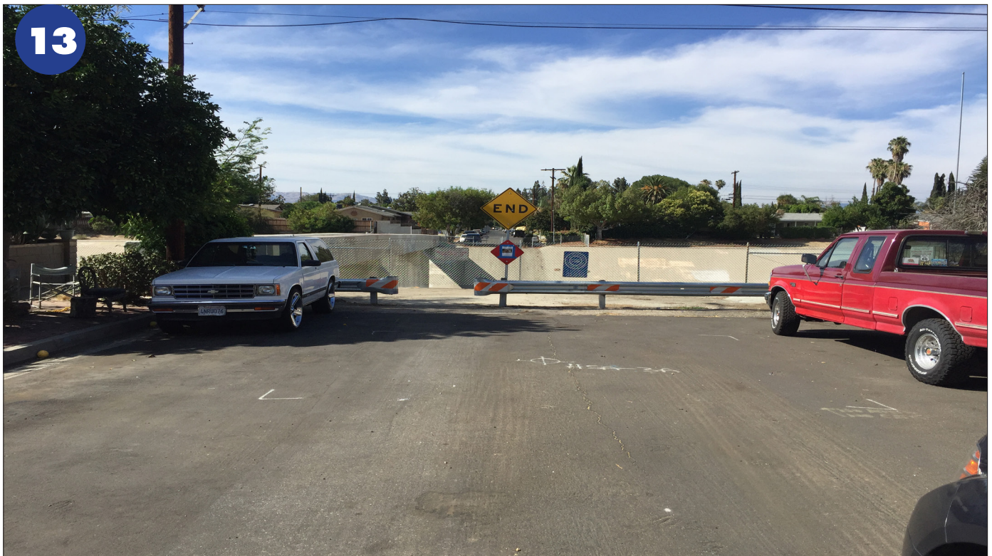
Amigo Street end, south bank of LA River, note lack of ADA-compliant access.
