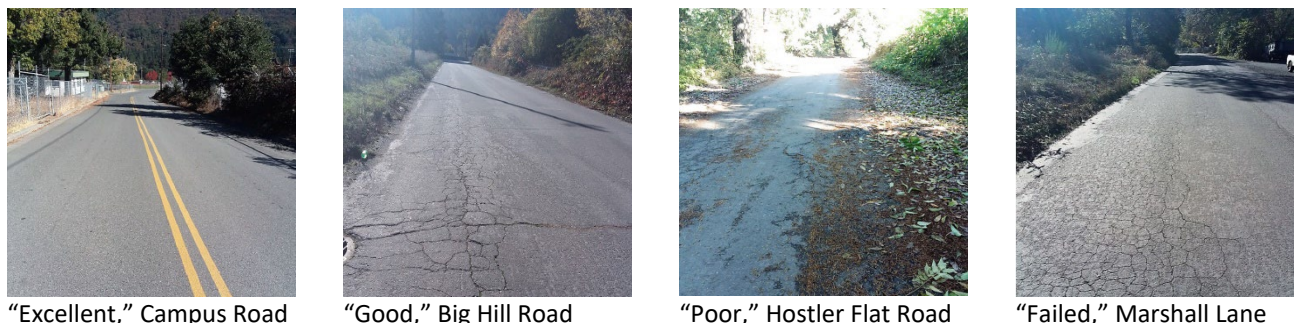
Figure 5. Examples of pavement conditions on tribal roads.
