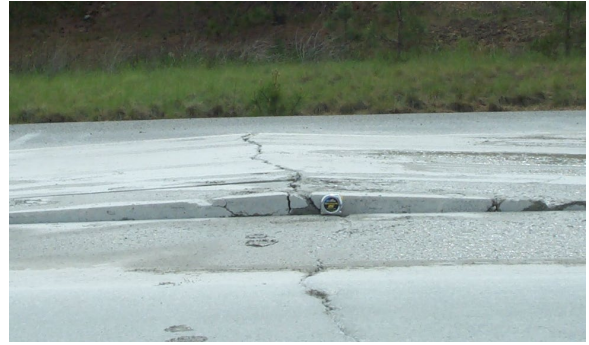
Figure C3. Example of concrete blowup.
