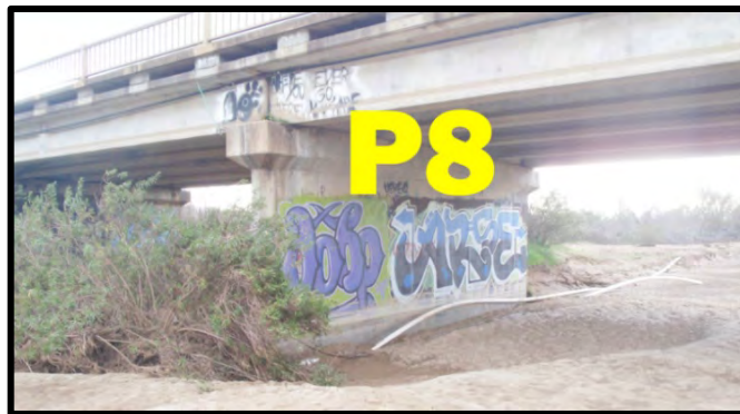
Two-foot scour hole at Pier 8, debris build-up and skew.
