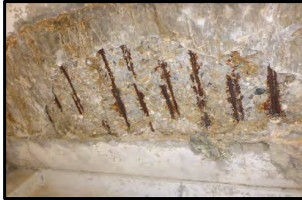
Typical soffit distress with exposed rusted rebar.
