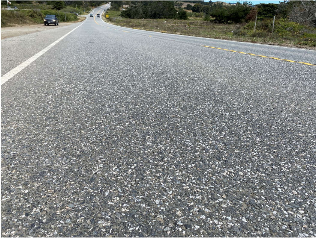
Figure 2- Pavement Condition at South of the San Gregorio Creek Bridge at State Route 001 @ PM 18.00
