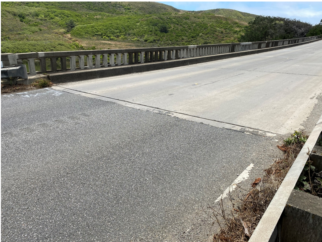
Figure 3- Pavement Condition at State Route 001 Approaching the San Gregorio Creek Bridge from South
