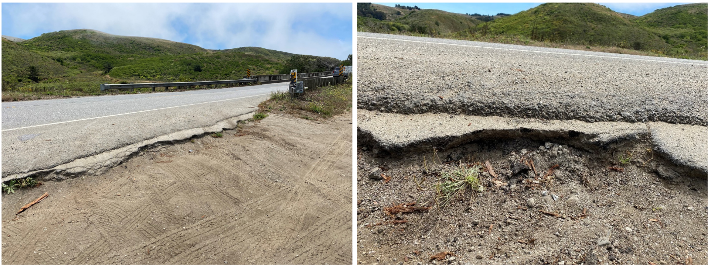
Figure 5- Pavement Shoulder Drop off at South of the San Gregorio Creek Bridge at State Route 001
