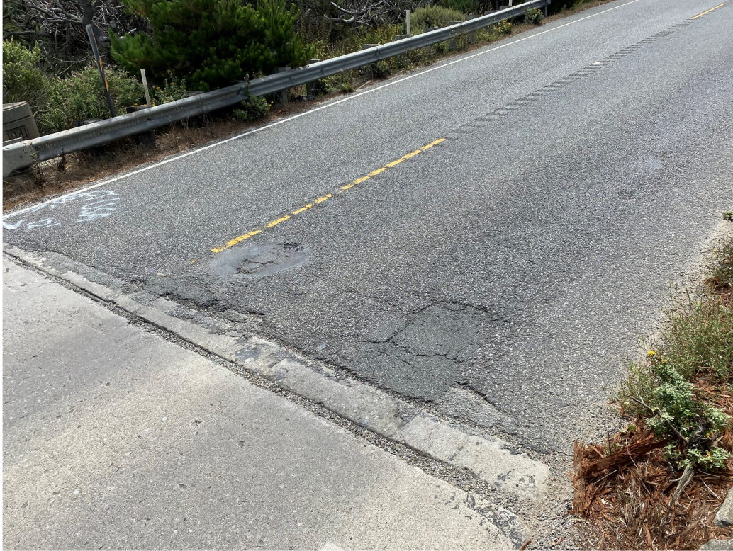
Figure 4- Pavement Condition at State Route 001 Approaching the San Gregorio Creek Bridge from North
