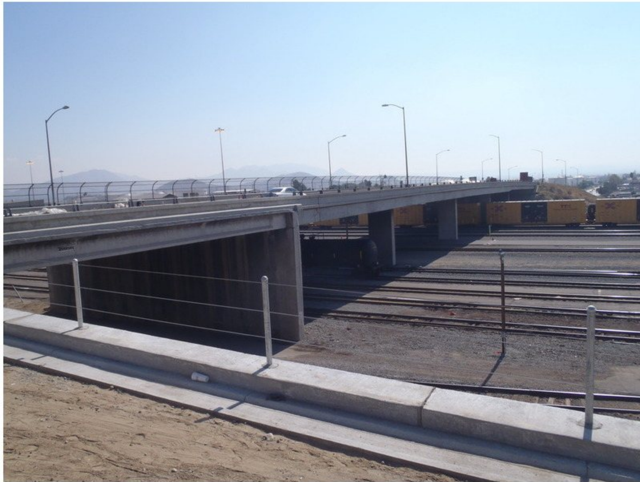
Photo No. 1 Routine elevation view looking south easterly from east bound offramp.
