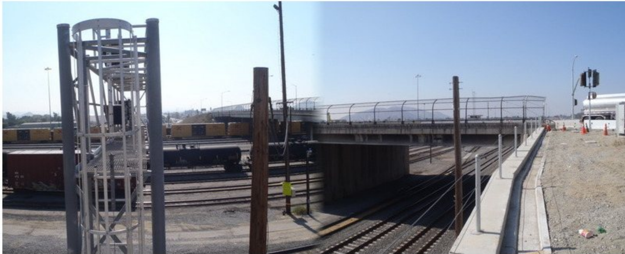
Photo No. 1 Panographic attempt at elevation view looking westerly. Railroad signal frame blocked view
